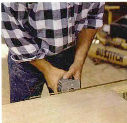
Trimming the edges flush. A laminate trimmer is just a router that's been downsized to make it more maneuverable. Here, the edge strip on the front of the countertop is being trimmed flush with the top of the substrate.
